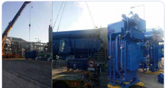
Hanhwa Chemical PE Manufacturing 1 Plant HWAR- L 1,400usRT(4,922kW)
