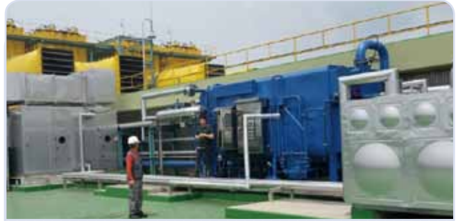
Korea Zinc. 2AA 210usRT(738kW), Air Handling Units Chilled Water Tank, Air Duct
