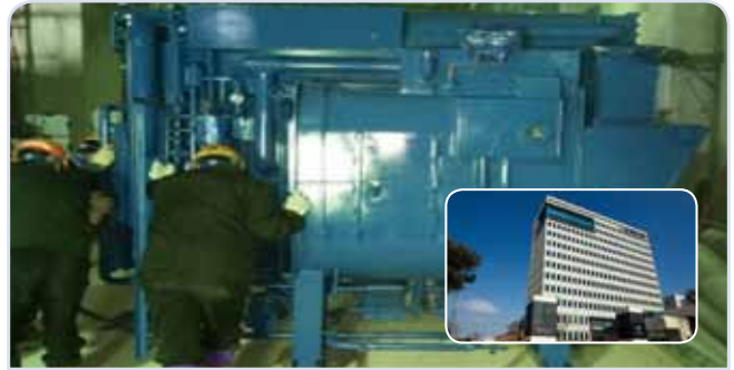
Korea Transportation Safety Authority Gimcheon Office DW 360usRT(1,266kW)
