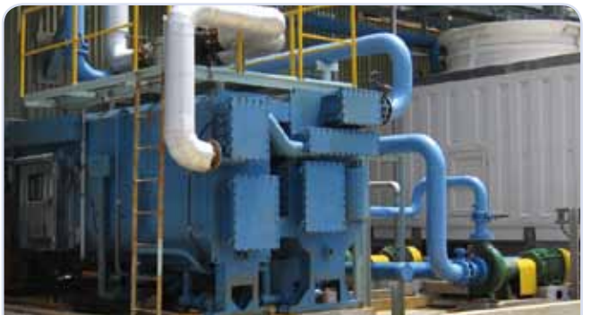
Youngpoong Seokpo Refinery 2AA 240usRT(844kW)
