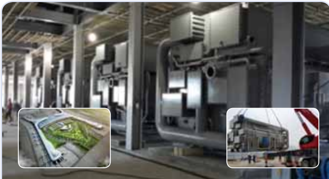
Incheon Interational Airport 2AB 8 sets 8,000usRT(28,128kW)
