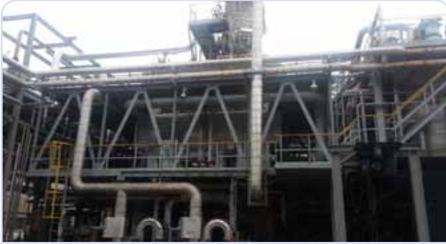
Kumho Petro-Chemical Factory HeatPump AHT (1.2barG Steam Production 8 ton/hour)
